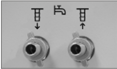
Fig. 72: Counter nuts on the cooling water nozzles
